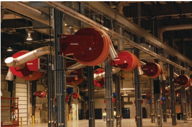
XL Hose Reels Installed and During Production, Fort Lee
